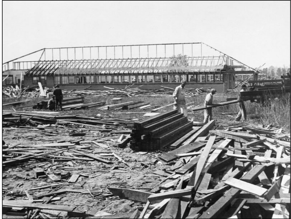
Figure 22. Dismantling of the Ross Field Balloon School for the construction of the Santa Anita Regional Recreational Center, 1932 (Los Angeles Public Library)
