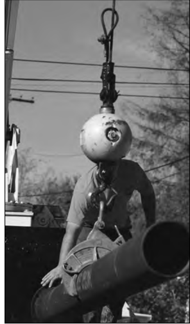
An Arcadia Public Works Services Department employee really puts his head into repairing a water main, 2000.
