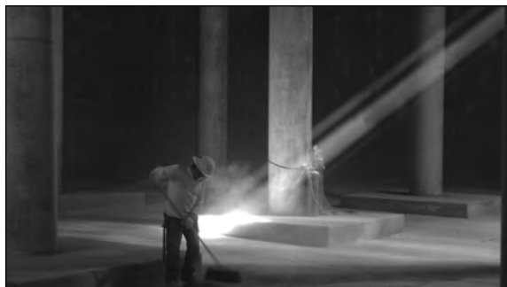
Arcadia Public Works Services Department employee removing last bit of dust in a new water reservoir, 2005.
