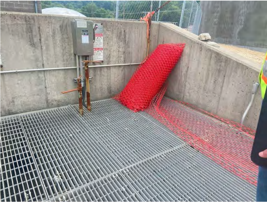
Figure 3: View of warped grating in back right section.
