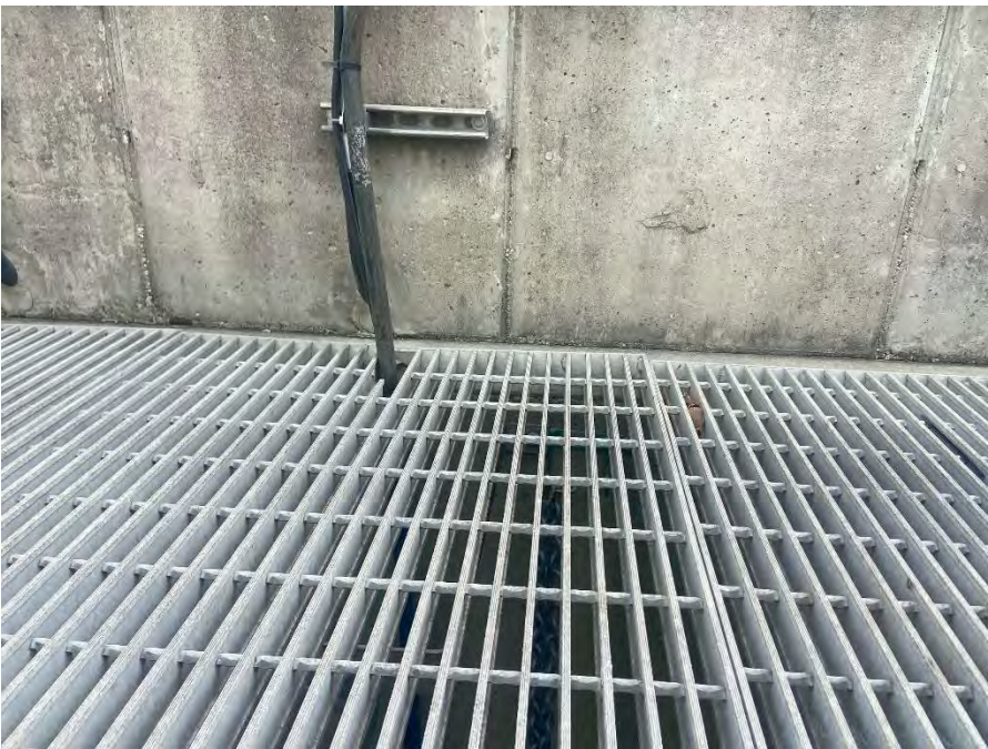
Figure 4: View of warped grating in back left section.
